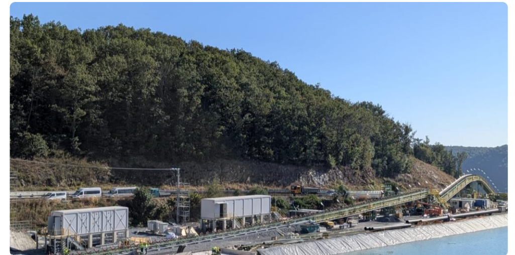
E-house and temporary genset
