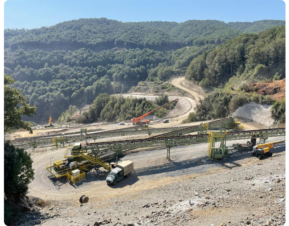
Filtered tailings conveyor installations
