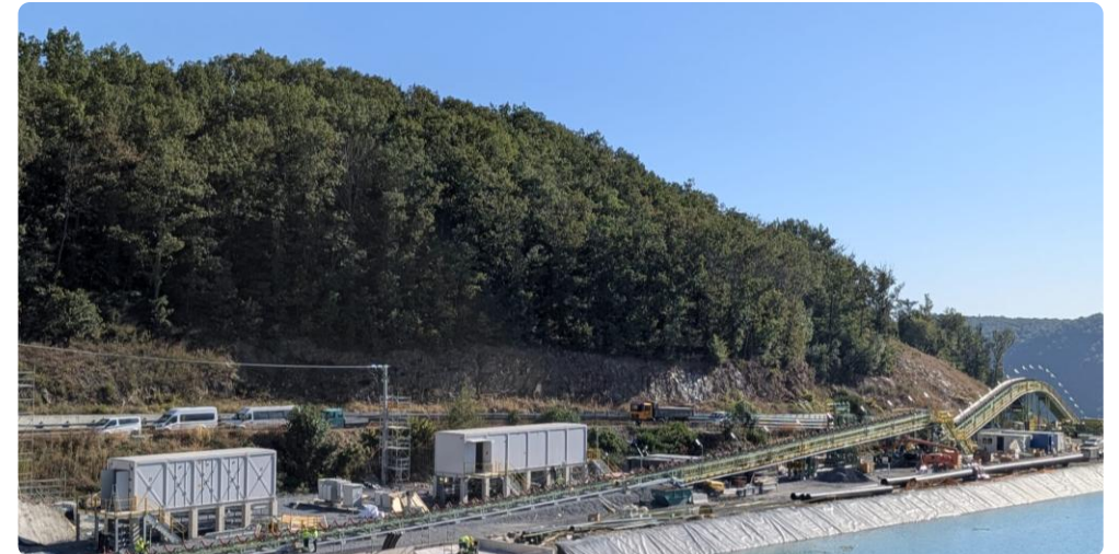
E-house and temporary genset
