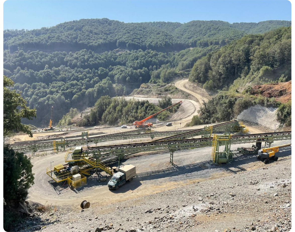
Filtered tailings conveyor installations
