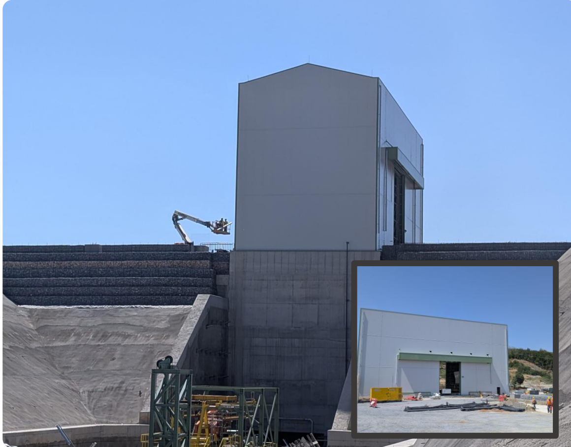
Primary crusher overview. Photo insert – Feed pocket
