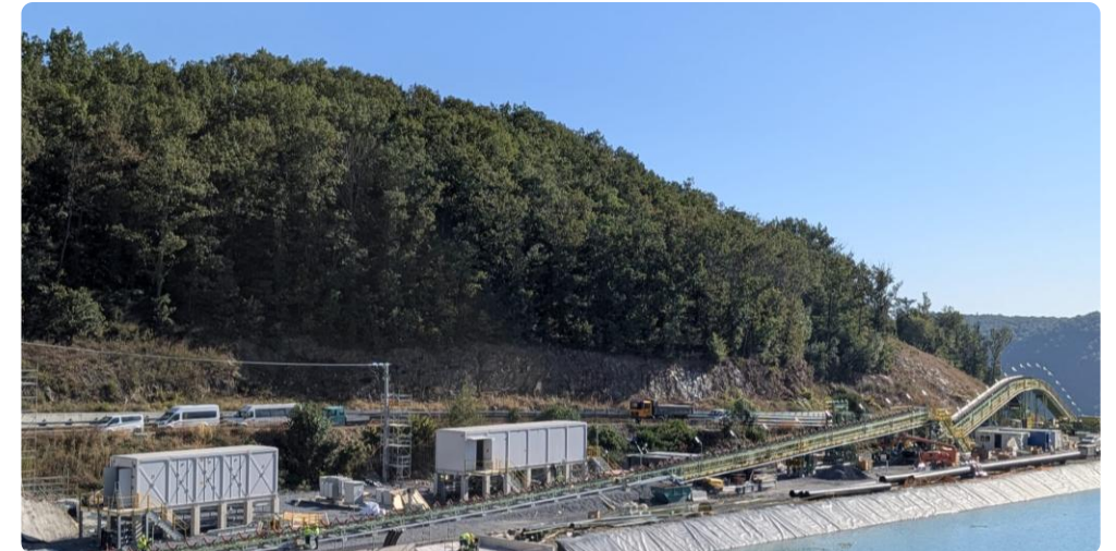
E-house and temporary genset
