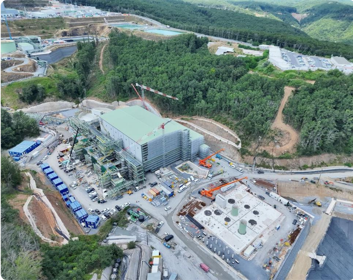
Filtered tailings plant overview
