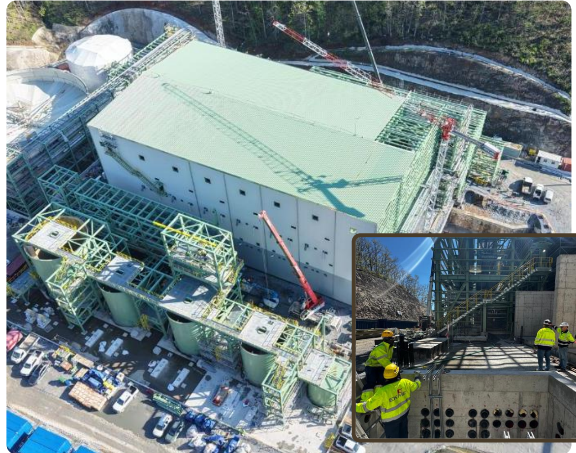
Tailings filter press building. Bottom right insert – closer up view of filter building pull pits.
