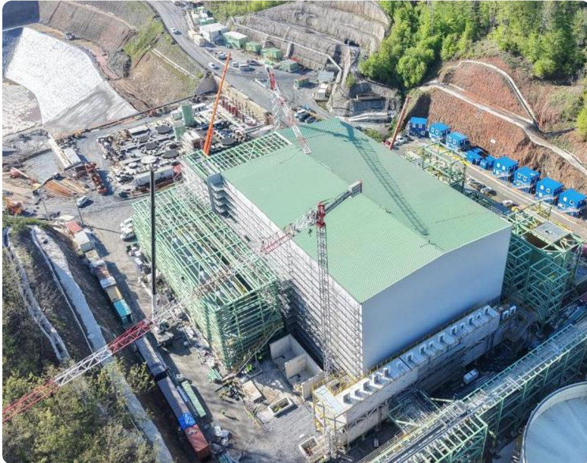
Filtered tailings plant overview, with tank farm progressing shown on the left and the foundation of the compressor building front right
