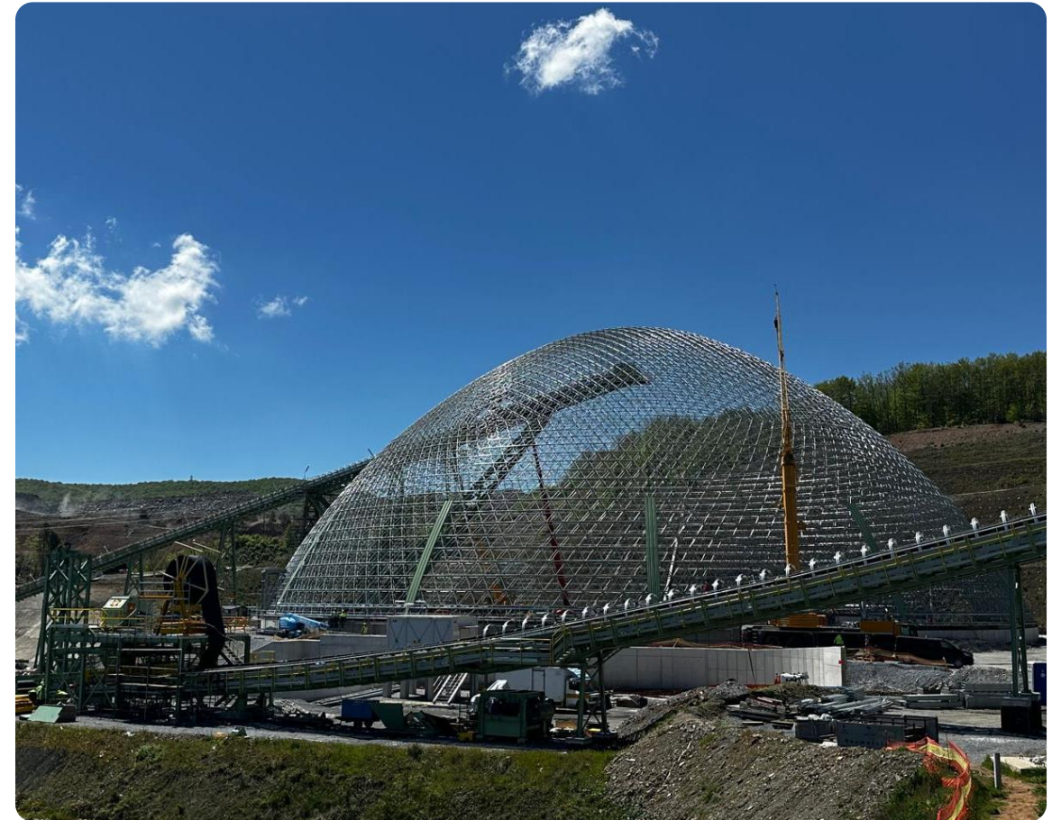
Dome and reclaim feeder, and dome, with SAG feed conveyor
