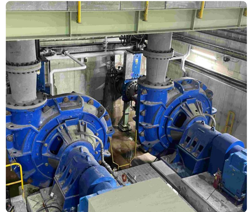
Cyclone feed pumps
