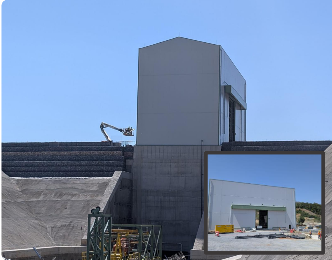
Primary crusher overview. Photo insert – Feed pocket
