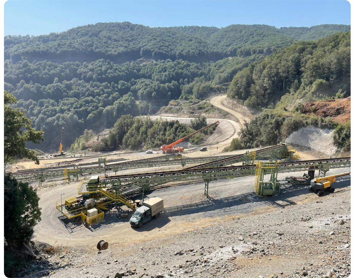
Filtered tailings conveyor installations
