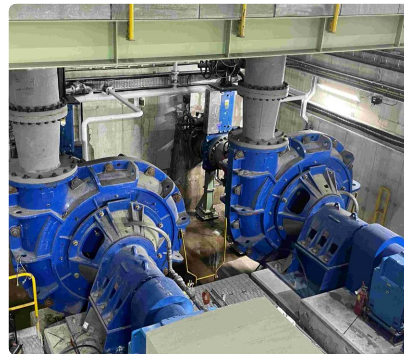
Cyclone feed pumps
