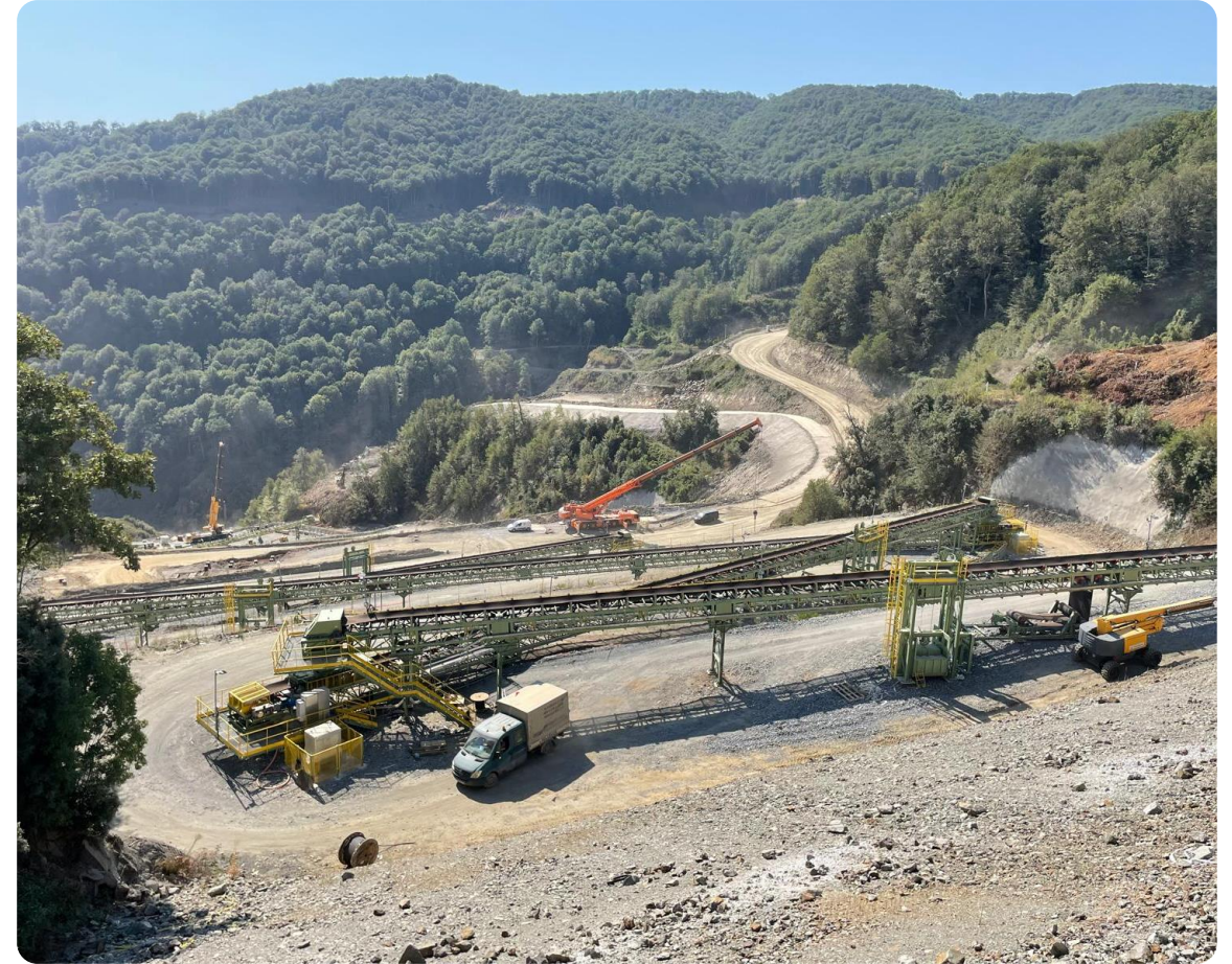
Filtered tailings conveyor installations
