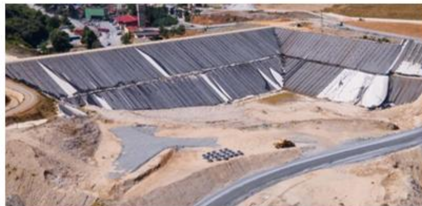
Triple-lined filtered tailings storage facility
