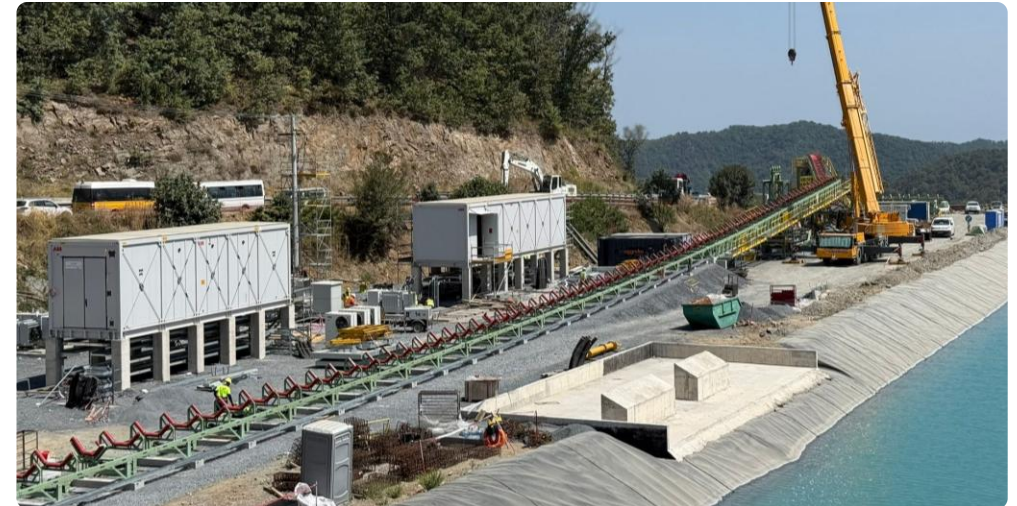
E-house and temporary genset
