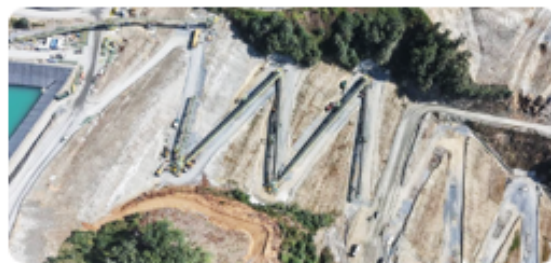
Overland conveyance system for filtered tailings to the dry stack facility
