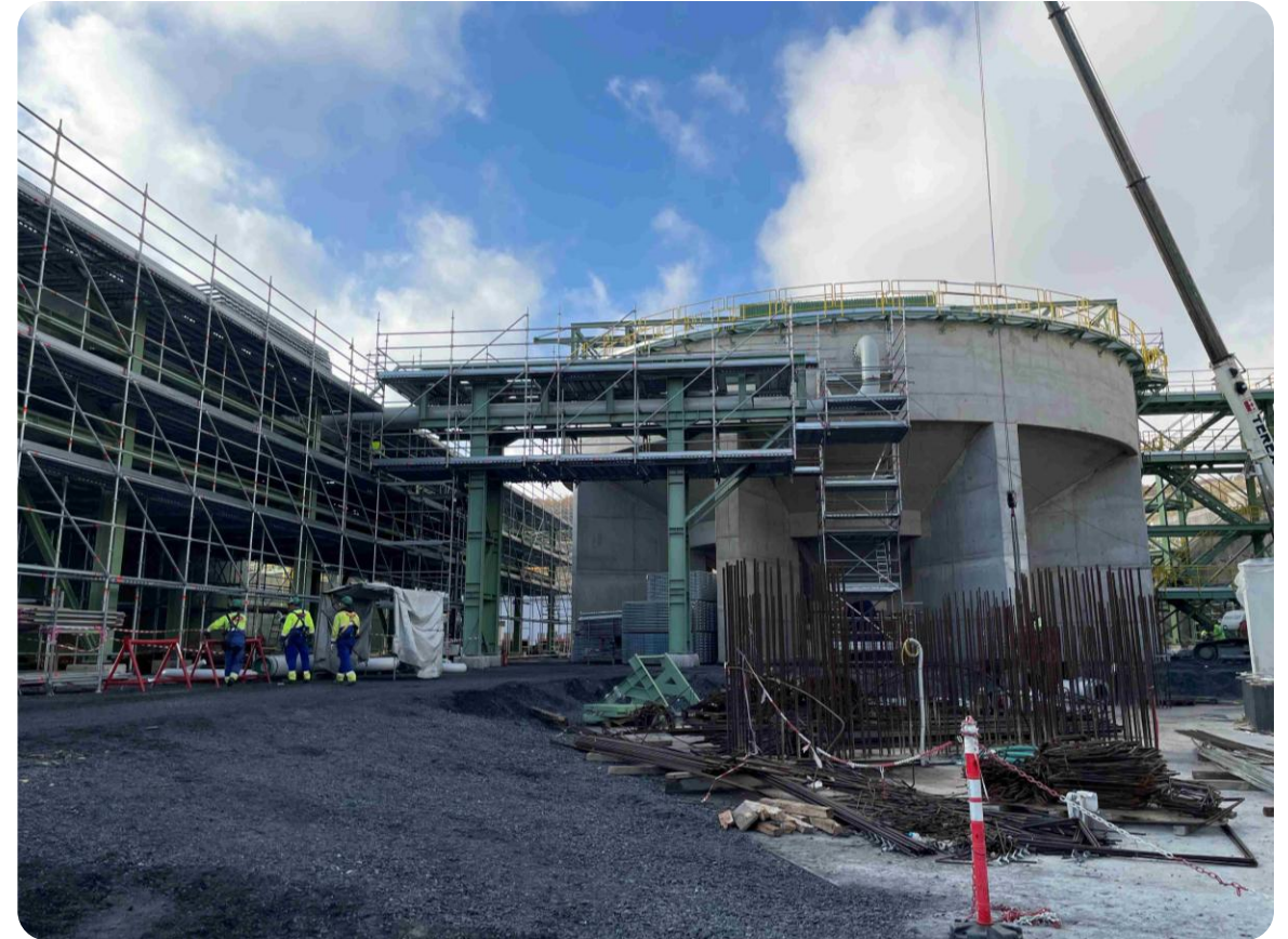
Tailing thickener pipe rack
