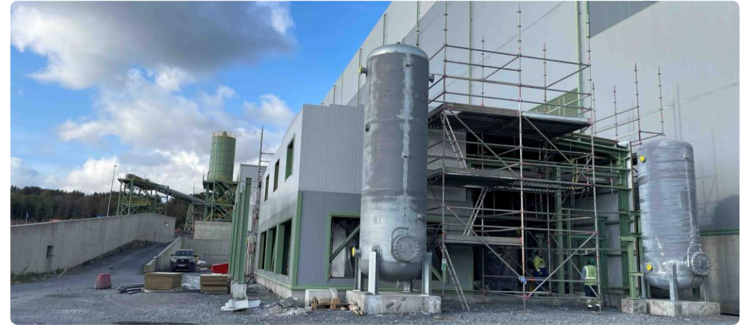
Process compressor building
