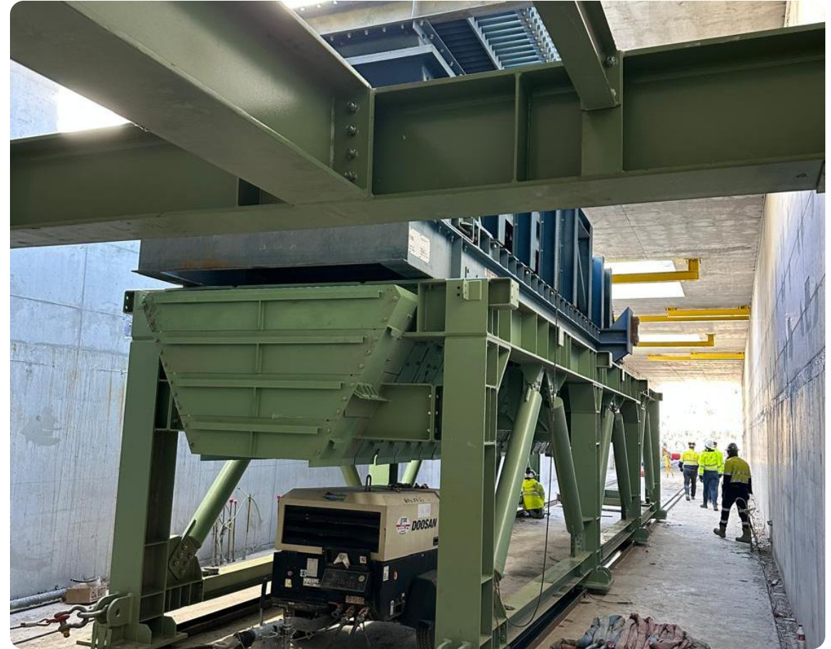
Reclaim feeder and discharge chute
