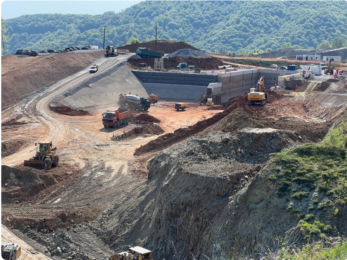
Excavations and slope stabilizations are progressing in all areas and the excavation and backfill for the conveyor alignment is in progress.
