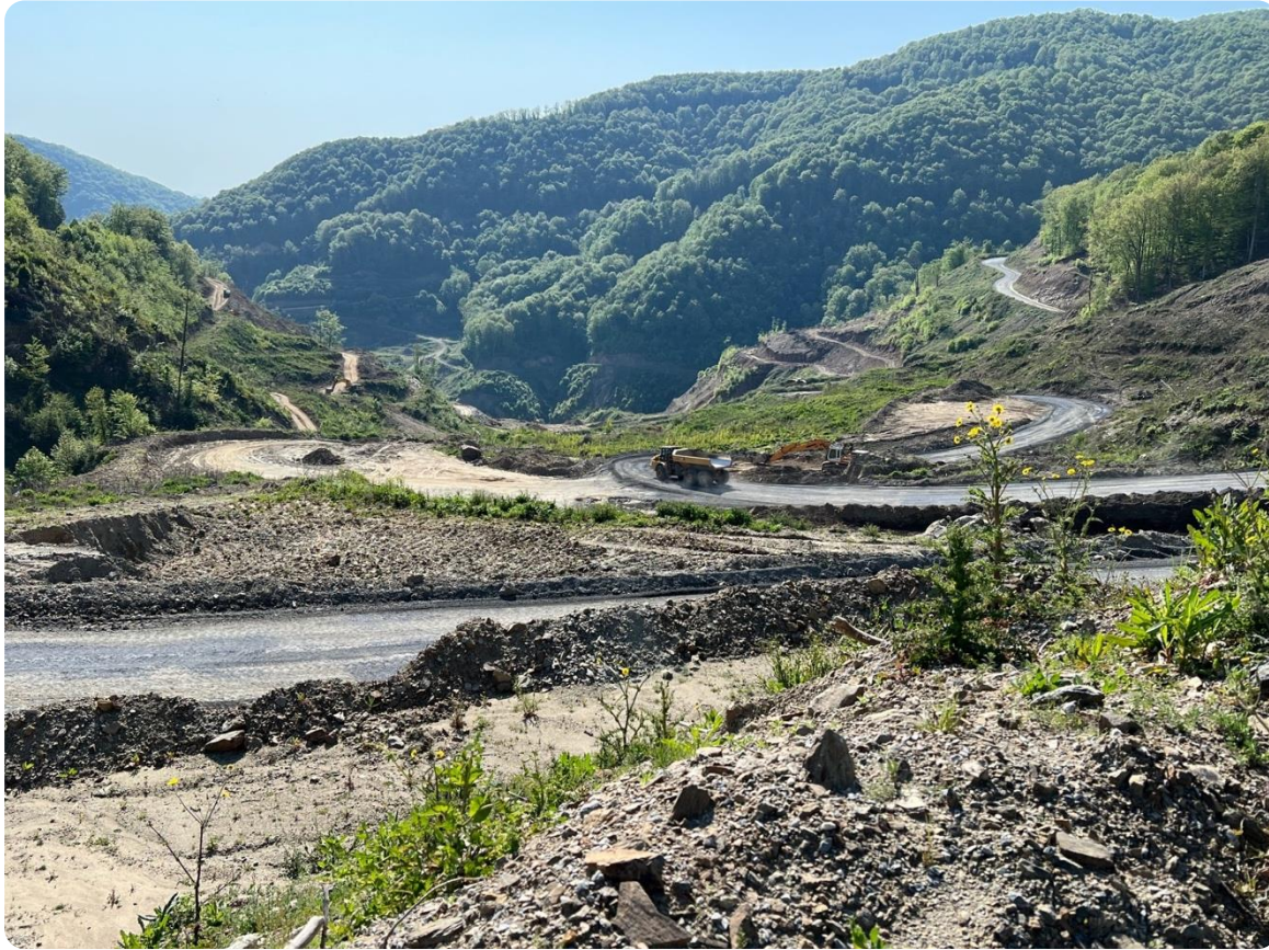
Low-grade stockpile area – currently excavating topsoil from the base of the low-grade stockpile.
