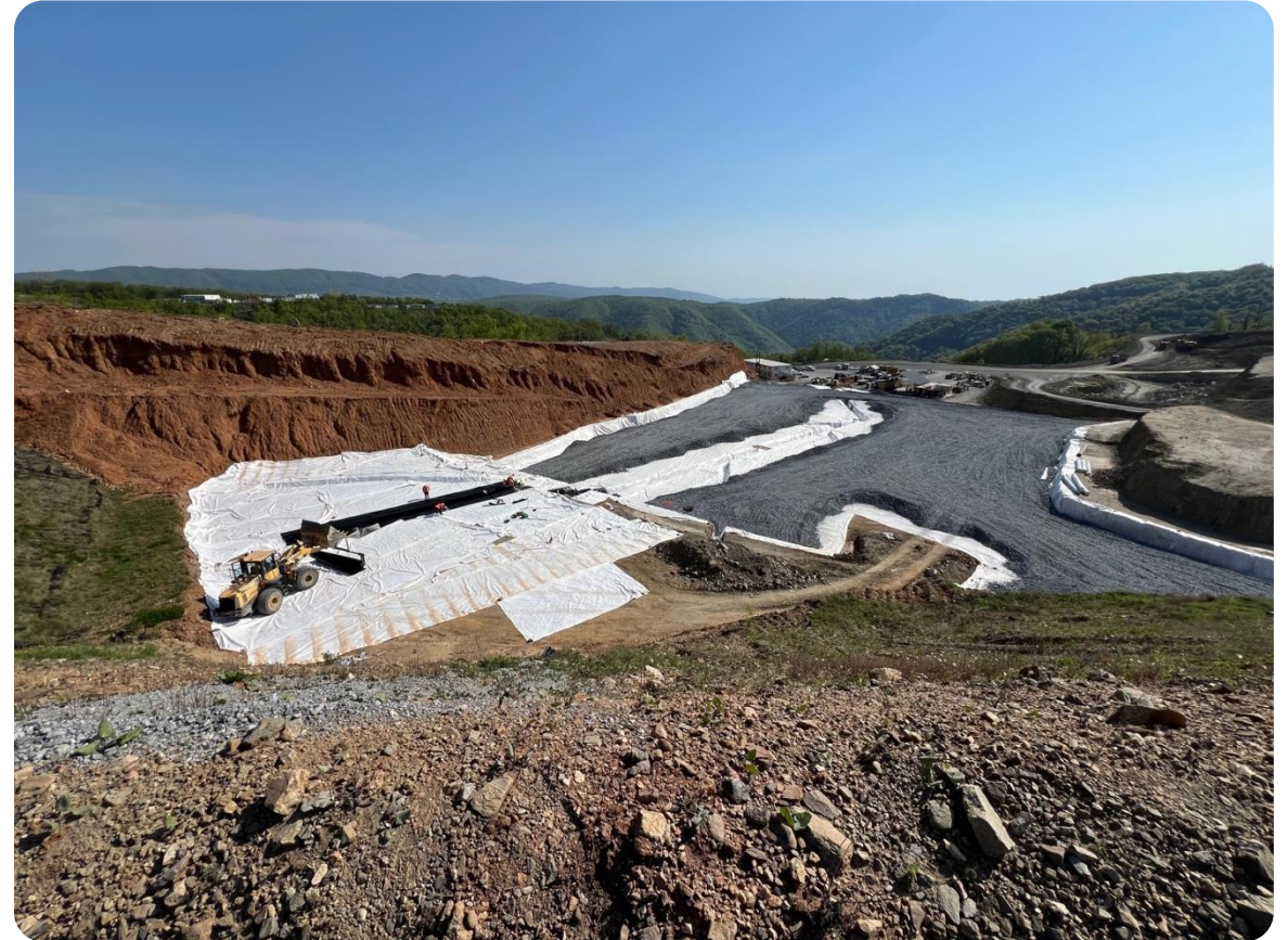
580 Pad – Geotechnical and Drainage Works prior to construction of OP/UG Workshops, Paste Plant and Warehouse.
