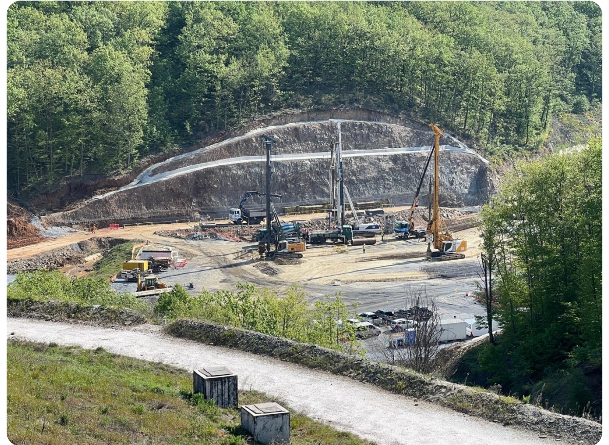
Four active drills are working at the filter plant, where 50% of the piles are completed (187 piles expected in total).
