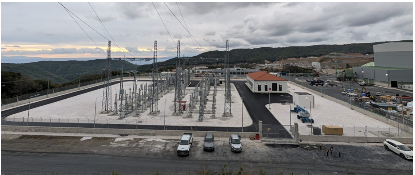
Process plant substation
