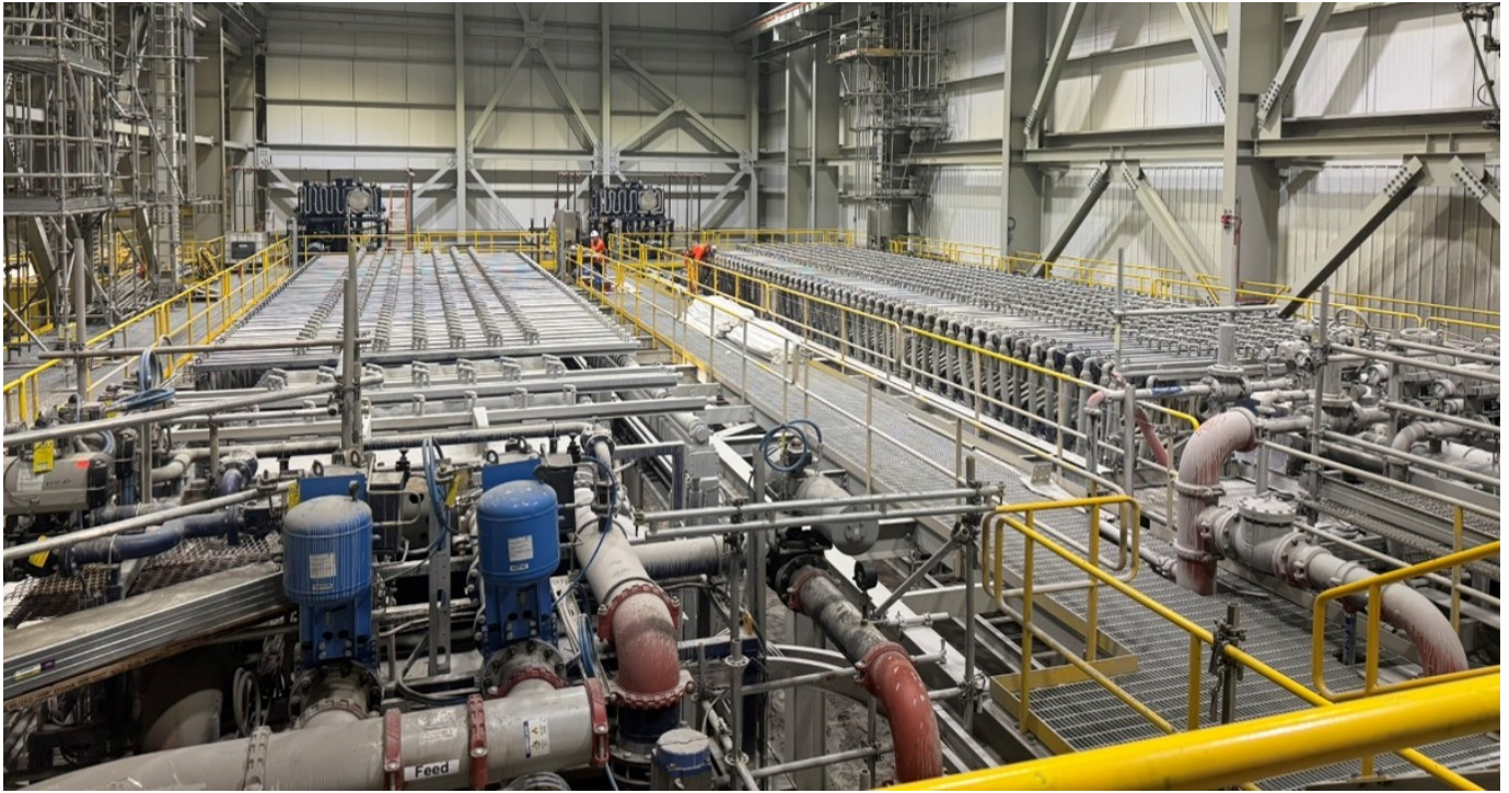
Tailings filtration within the process plant
