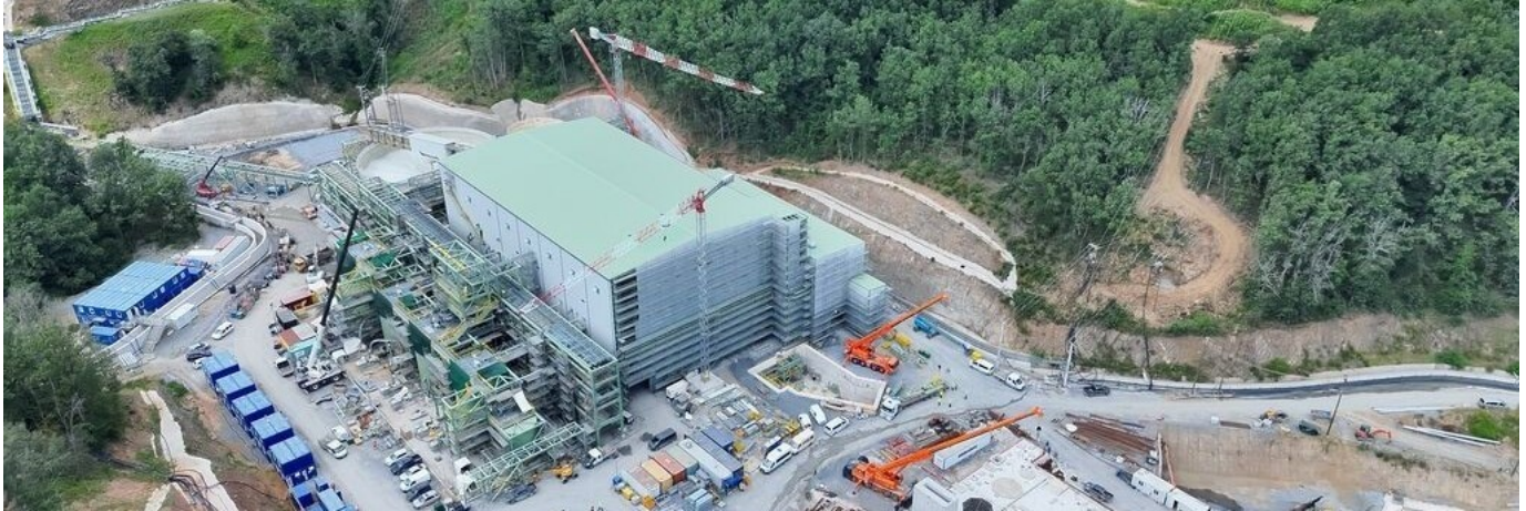
Filtered Tailings Facility
