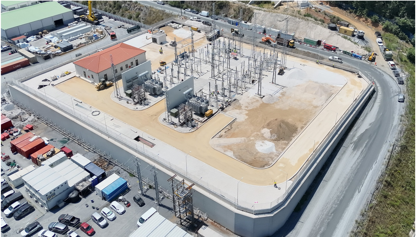
Process plant substation
