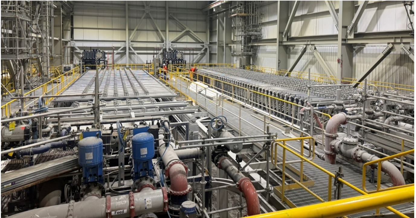
Tailings filtration within the process plant
