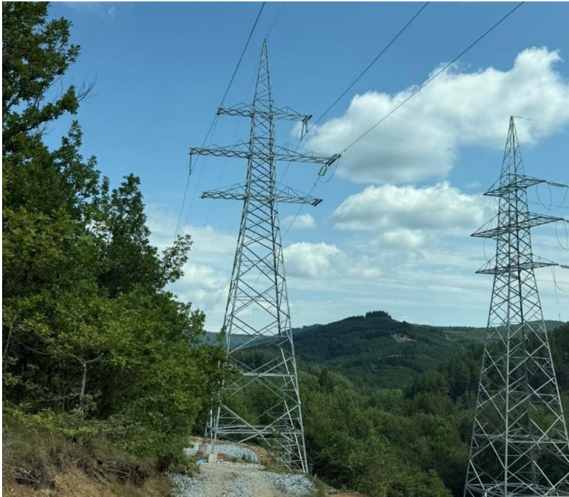
Final transmission tower
