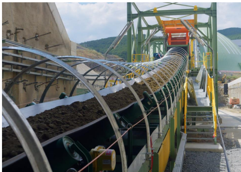
Crushed ore conveyed from the primary crusher to the coarse ore stockpile
