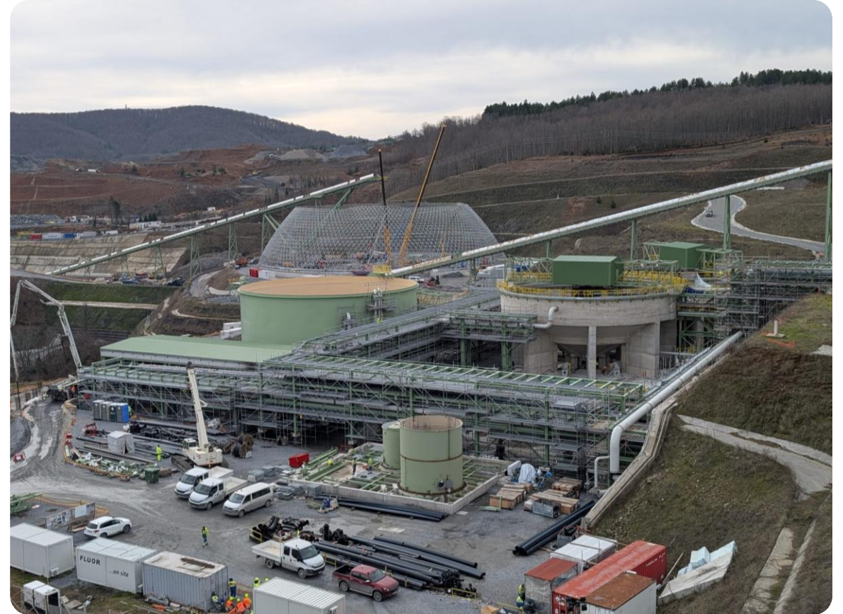
Tailing thickener pipe rack and distribution box
