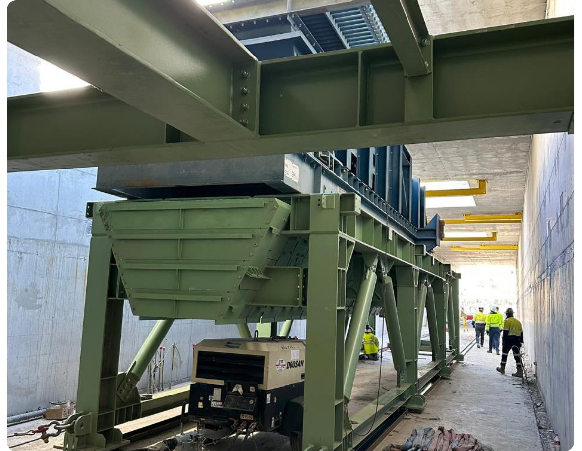
Reclaim feeder and discharge chute
