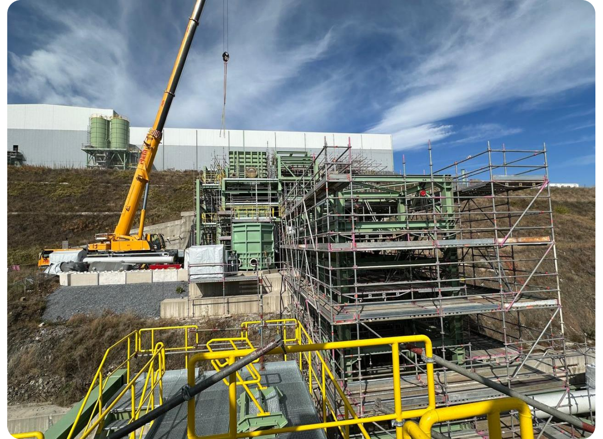
Tailing thickener pipe rack and distribution box
