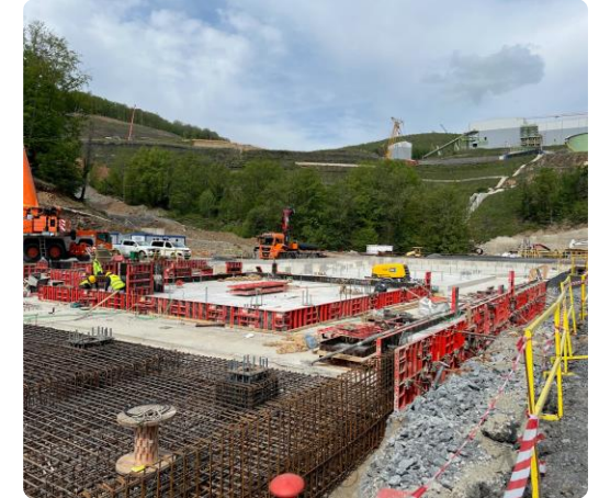
Tank farm bases
