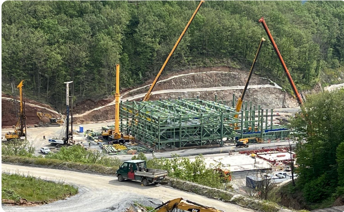
Filtered tailings plant facility overview
