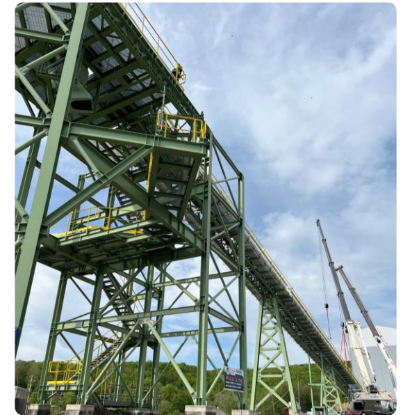
Conveyors from the pebble crusher to the transfer tower
