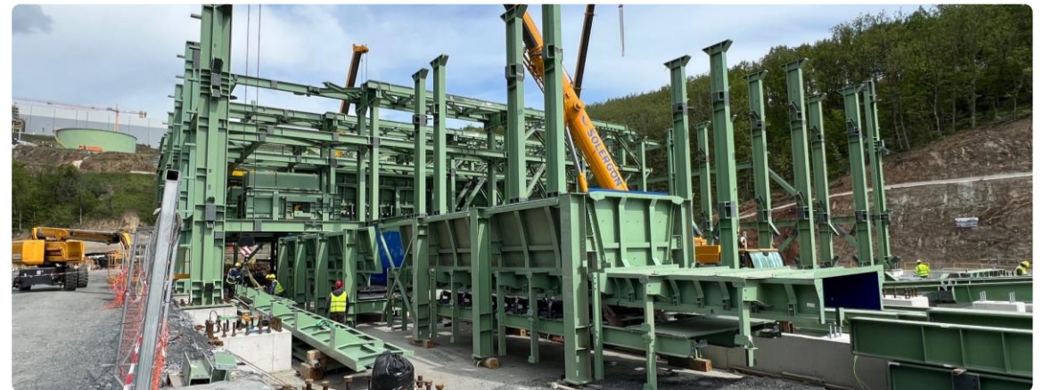
Filtered tailings building– close-up view of the structure, including the feeder conveyor
