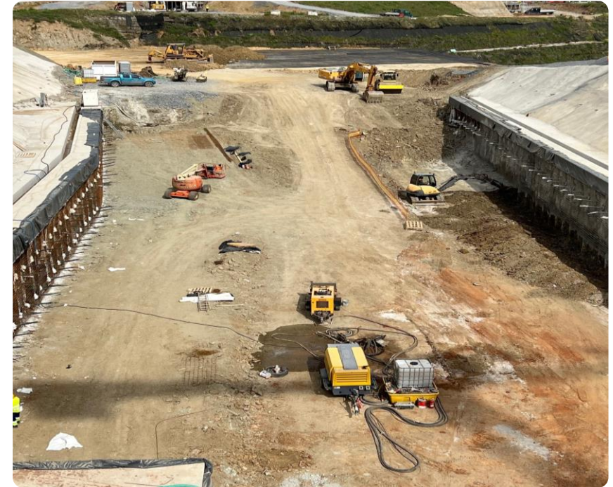
Primary Crusher – conveyor alignment
