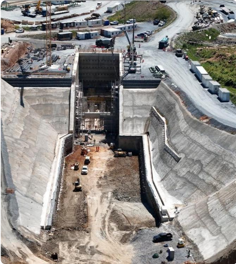
Primary crusher overview
