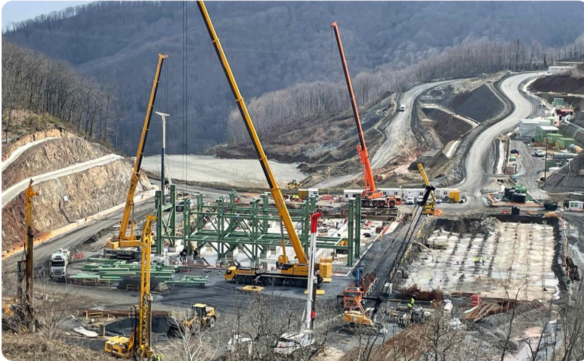
Filter plant facility overview – February 21, 2025
