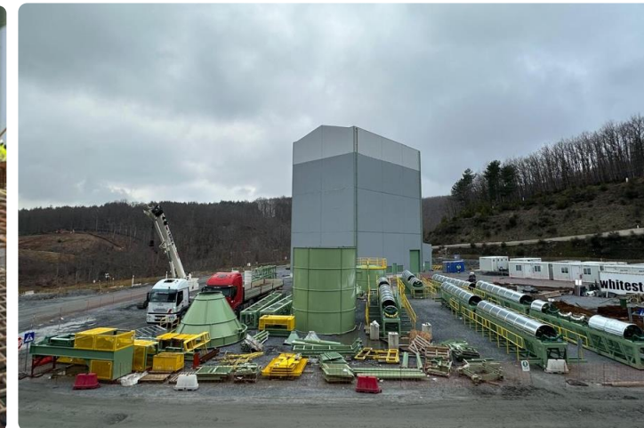
Conveyors and lime plant platework
