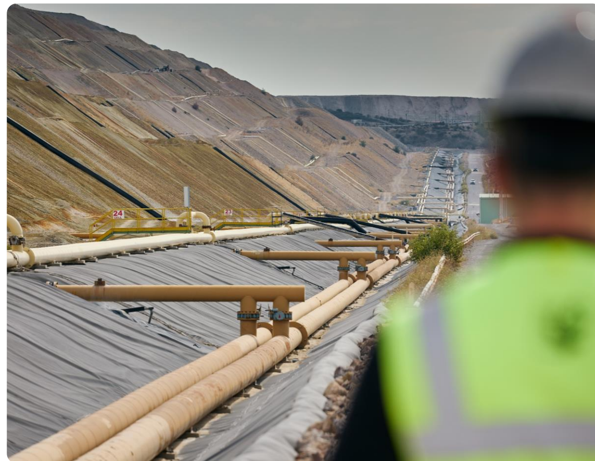
Heap leach solution recovery infrastructure at Kışladağ.
