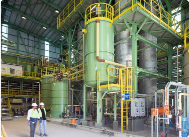
Top: Aerial view of North-ADR plant and infrastructure; Bottom: Interior of North-ADR plant.
